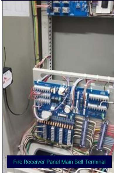
Fire Receiver Panel Fire Contact Point
